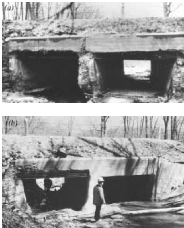
Fig. 1.5—(a) Deteriorated double-box culvert showing advanced deterioration and distress before repair; and (b) concrete in culvert restored with shotcrete with natural or gun finish.
