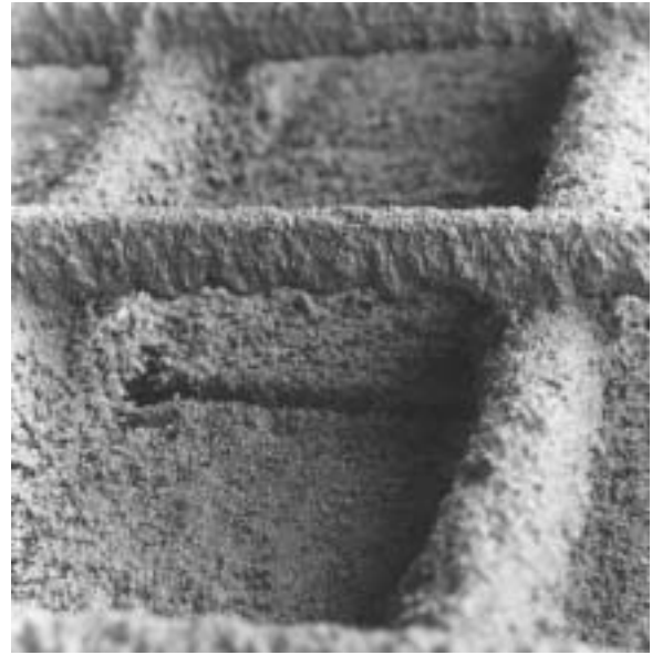
Fig. 8.10—Overspray on reinforcing bars at the top of a band of shotcrete.
