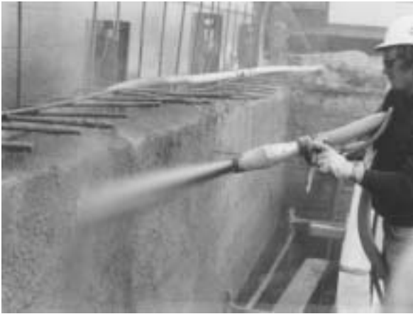
Fig. 8.7—Dry-mix shooting final coat of 1 to 1-1/2 in. (25 to 38 mm) of shotcrete to previously gunned wet shotcrete base.
