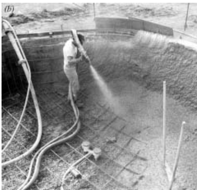
Fig. 1.3—Applying wet-mix shotcrete: (a) as scour protection to a spawning channel; and (b) in a swimming pool.
