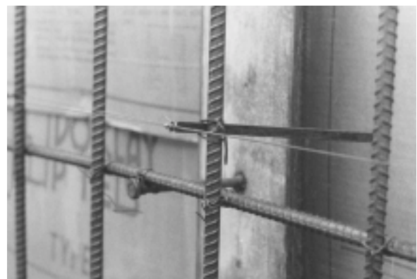
Fig. 5.5—Ground wire attached to depth gauge, which is tied to reinforcing steel and will be left in place.
