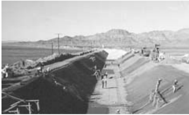
Fig. 1.2—Dry-mix shotcrete lining being installed in a large water irrigation channel in Arizona.
