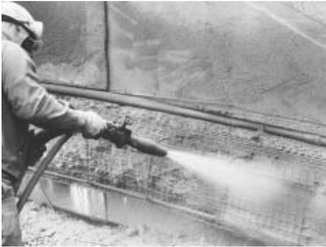
Fig. 5.2—Shooting through welded-wire mesh cut and bent to follow contours or repair.
